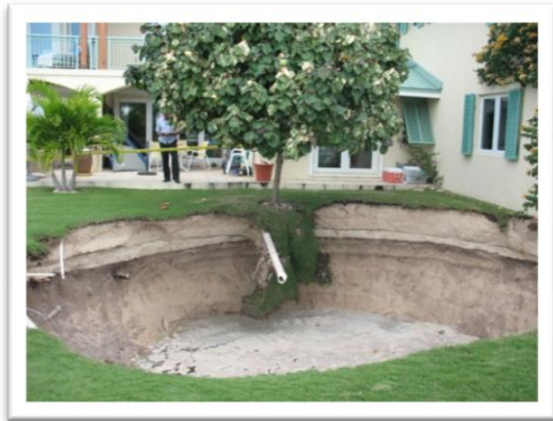
Sink Hole at Pirates Point 3
